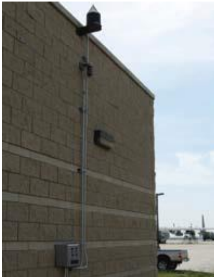
The maintenance building with controller, rain gauge, and alarm light.
