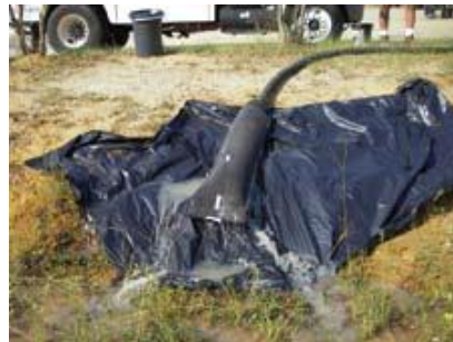
EVAC Filter is attached to a hose from the frac tank. The water is filtered to a non-detect level for hydrocarbons.
